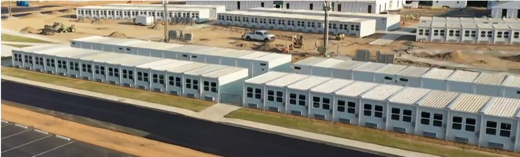
In Wynne, AR, we delivered 180 flex modules for the Wynne School District within 90 days following a tornado. We are uniquely positioned to rapidly deploy large complexes for any flexible space need.
